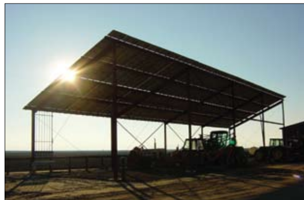
Fixed Solar Panels
